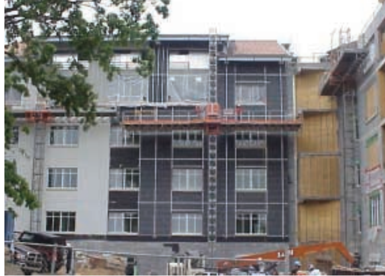
Companies are slowly returning to mast climber rental in the UK, albeit with a different offering, with at least four companies now covering the market place.
