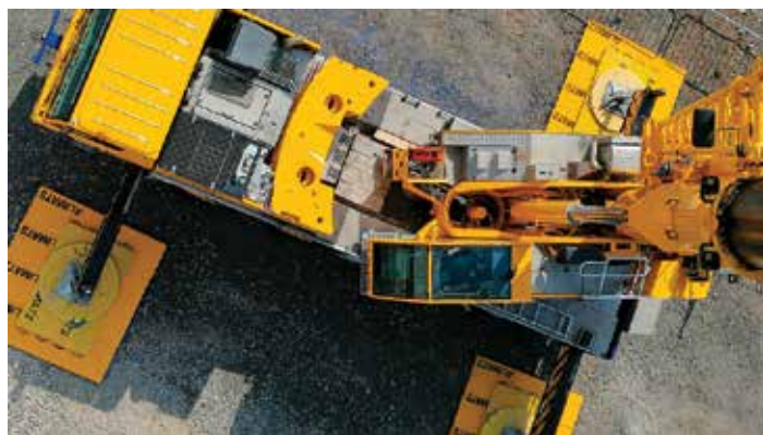
A new Dingli BT24ERT lithium boom lift from Clements and a Demag AC60-3 from Aba Crane Hire working on Warwickshire's Chesterton Windmill using aluminium trackway panels to gain access
