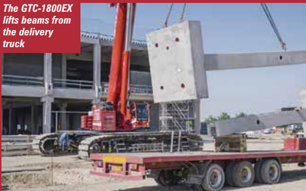
With slings replaced by a lifting rod, the beams are turned to the vertical...
