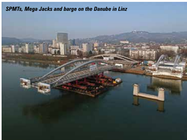
The 50 metre bridge section for the new Seibert Bridge is loaded onto the barge
