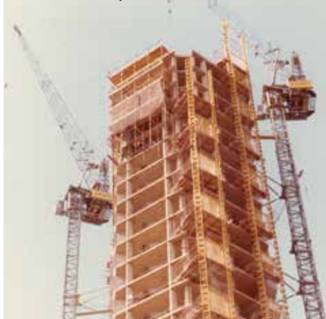
Three of Laing's 50HBs were used to build the Penta Hotel in Cromwell Road, London
