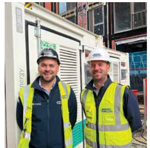
Senior site manager Charlie Falkingham (L) with assistant crane manager Tom Carter on site with the AMPD Energy battery energy storage systems
