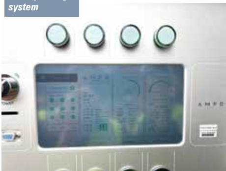
The control panel on the AMPD Energy battery storage system
