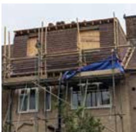
The unsafe scaffold
