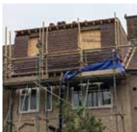
The unsafe scaffold
