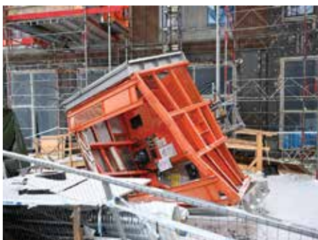
Five occupants in this hoist car died when it crashed to ground from a height of around 20 metres
