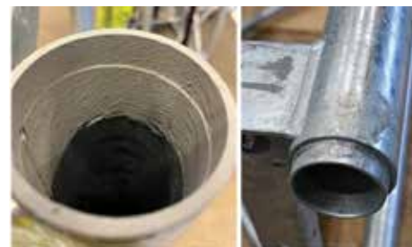
With critical bolts missing, the mast sections were only held in place by the friction between the short spigots and the sockets of the section below
