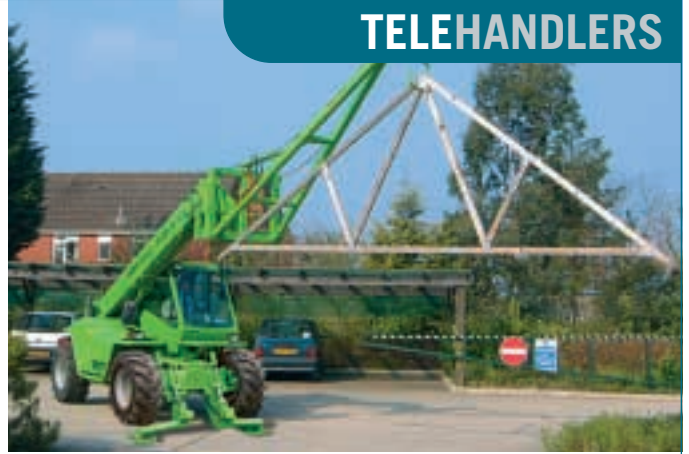
Merlo has introduced attachments specifically designed to permit its telehandlers to travel with the boom lowered while transporting roof trusses on site.
