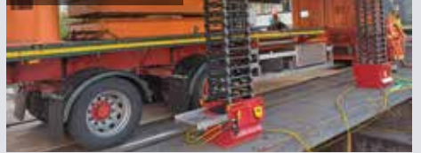
Bridge deck rotation completed, Enerpac cube jacks lower the bridge onto the flatbed trailer
