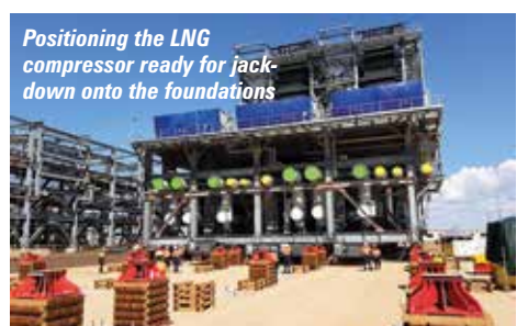
One of the Enerpac EVO power packs used to operate 24 jacks to lower the load onto pre-prepared foundations
