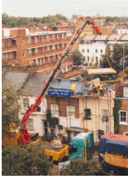
Paul Hare of Hare Home Improvements says that the company has been able to abandon the use of fixed jib cranes and use a specially developed Mercedes/Fassi F420AXP.26 knuckle boom with the latest generation remote control
