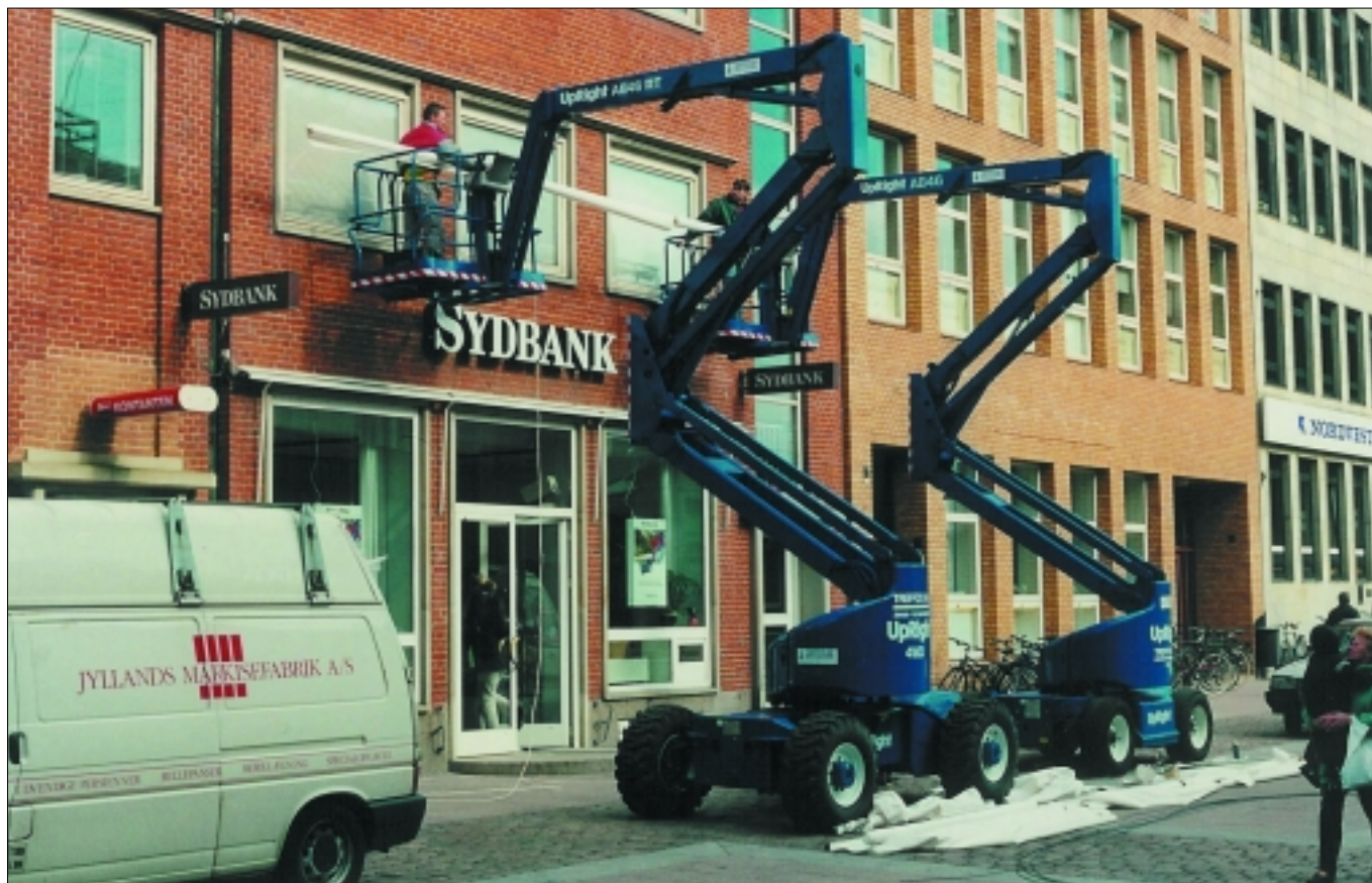
UpRight's AB46 has an outreach of 8 metres, aided by a 1.5 metre jib. Pictured are two units supplied by UpRight's Danish distributor, Treffco for the installation of a sun guard on a city centre bank in Aarhus
