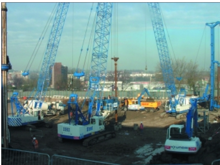
One of AGD Rental's 70 tonne capacity IHI DCH 700 heavy duty piling cranes being assisted by two, 50 tonne capacity IHI CCH 500 handling cranes
