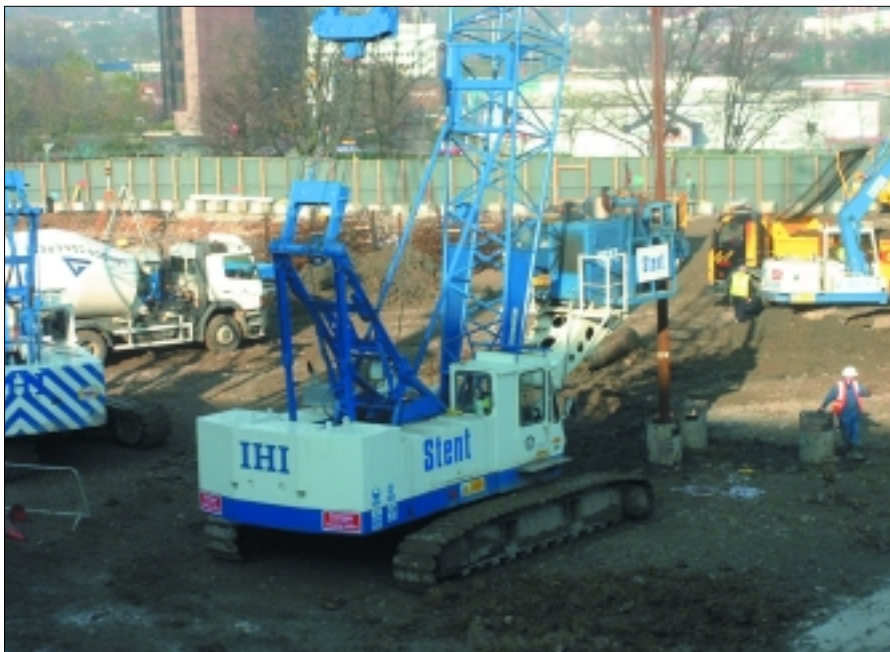
Part of the long term rental contract between Stent Foundations and AGD saw AGD's equipment painted in Stent's blue and white livery. Pictured is one of AGD's IHI DCH 700 piling cranes fitted with one of Stent's Watson piling rigs
