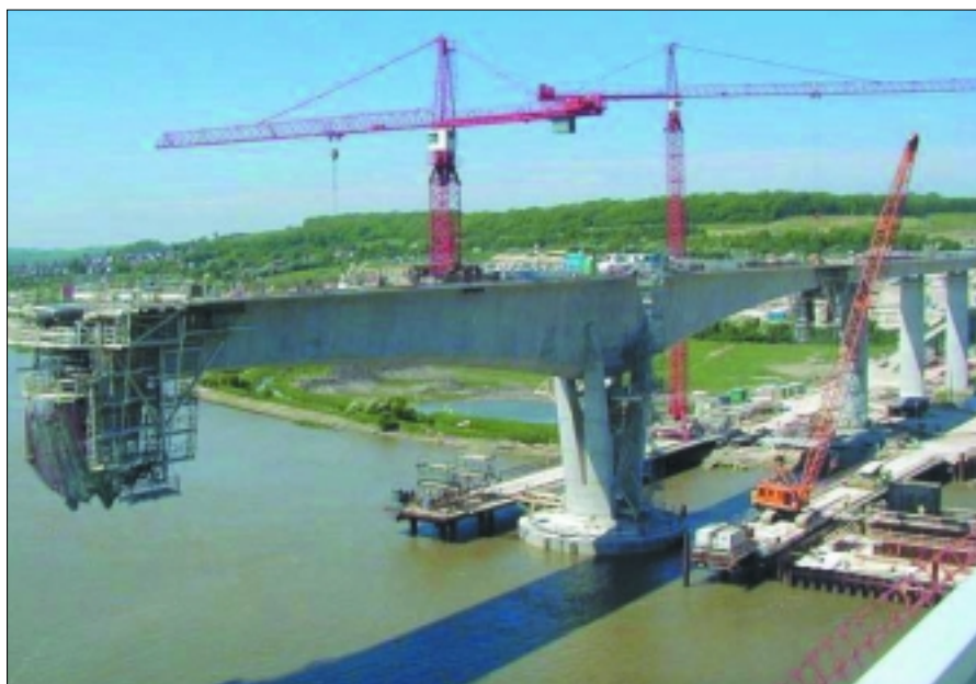
Kier Plant and Arcomet designed and fabricated special steel bases for two rail-mounted tower cranes on the permanent deck of the Channel Tunnel Rail project at the Medway Crossing in Rochester. A further two towers have been erected on temporary 80 metre long jetties.
