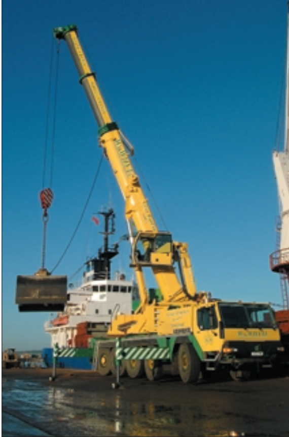
The Liebherr LTM1100/2 with telescoping elevated cab the livery of William Whyte of NE Scotland
