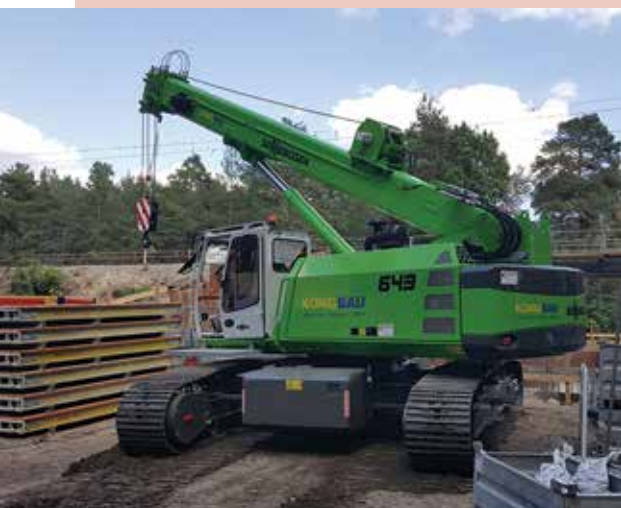
König Bau using a new Sennebogen 643 telescopic crane is used for a variety of lifting tasks.
