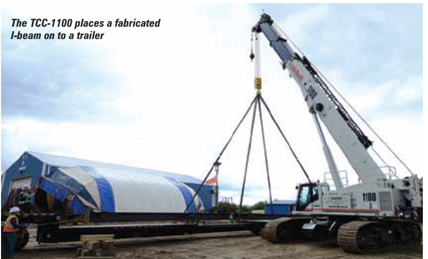
The 100 tonne Link-Belt TCC-1100 and 90 ton HTC-8690 truck crane tandem lift a 20 tonne metre skid at Davco's yard in Wainwright
