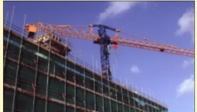
A rare sight in London is this BPR GT215B tower crane belonging to Falcon Crane Hire which has been erected on the Chrisp Street site in Poplar to lift a variety of structural components, building materials and equipment for Durkan Construction and its sub-contractors. BPR was an independent French crane builder which became part of the Potain group some years ago. This particular model has been retrofitted with an Smie AC30 electronic control system from Cranesafe Limited to prevent it oversailing the nearby Docklands Light Railway. Falcon Crane Hire has nine Smie AC30 systems installed on a variety of cranes.
